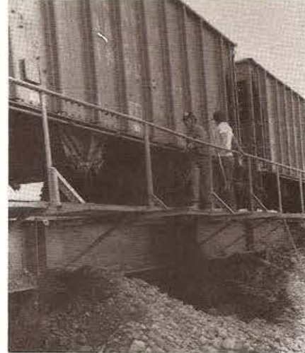
Close-ups of cars being unloaded and gravel moving over the conveyors on the jobsite. An operator mans remote hydraulic hopper gate controls which can shut off the flow of gravel to the conveyor belts if problems arise.
